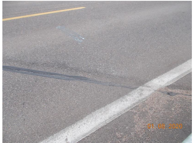
Suspect asbestos-containing material M-22-U-TR01. The tar expansion joint material is non-detect for asbestos.
