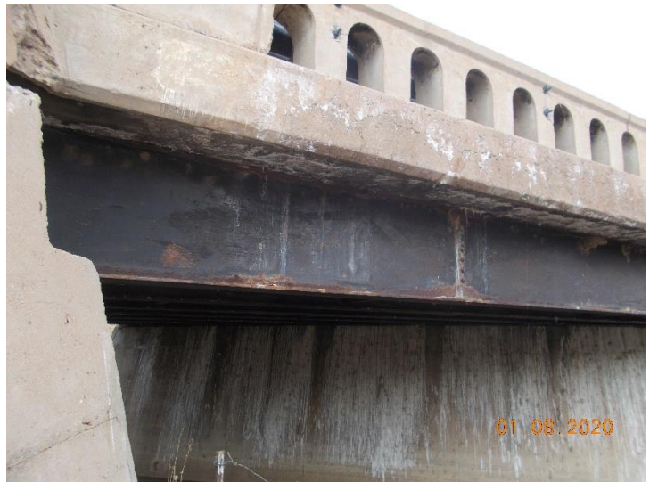
Paint sample M-22-U-LP02. The black paint on the metal girders is considered lead-based paint.
