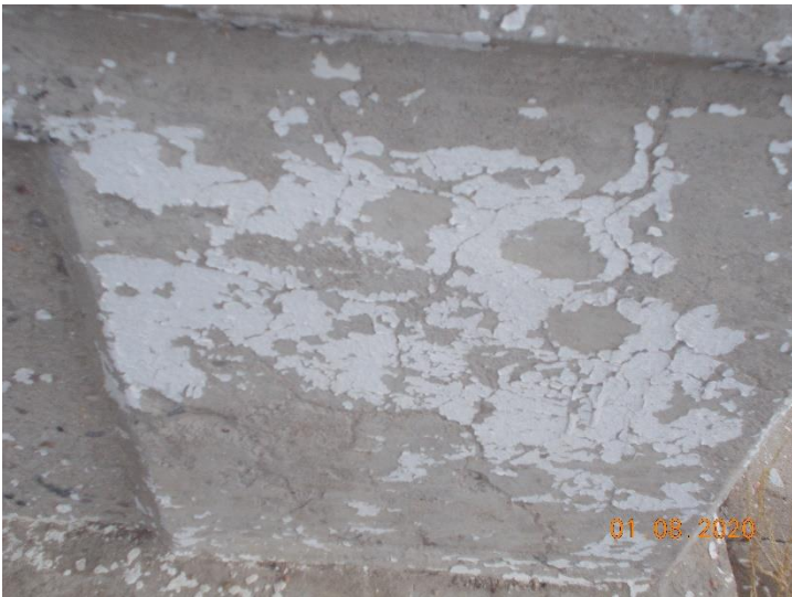
Paint sample M-22-U-LP01. The white paint is considered lead-containing paint.
